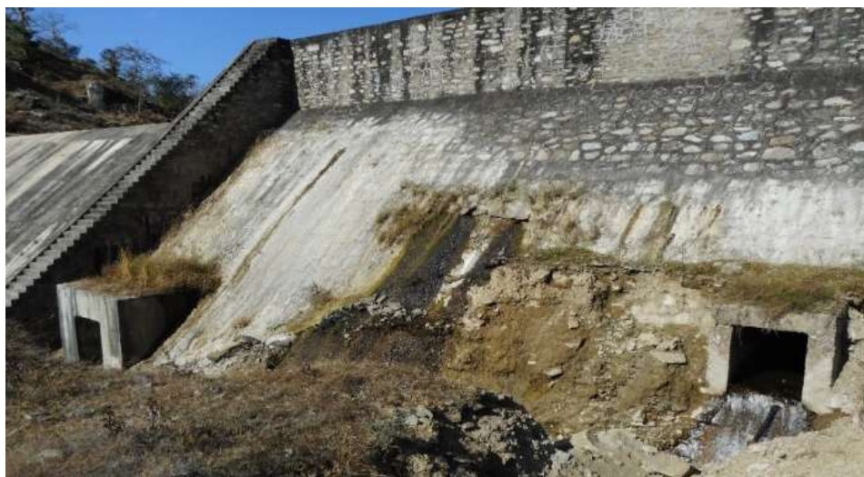
Leakages in the Rohini dam
