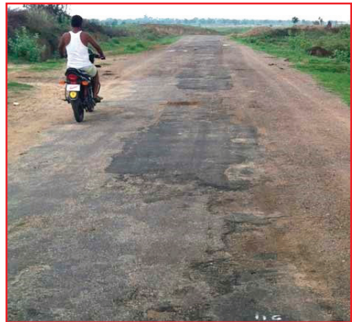
Figure 9: Road surface showing a history of routine maintenance, now due for resealing
