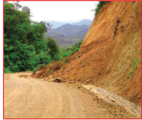
Figure 10: Emergency maintenance required for landslide
